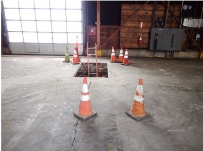
SLAB OPENING CREATED AT LOCATION OF PUNCHING FAILURE DUE TO DROPPED STEEL COIL
