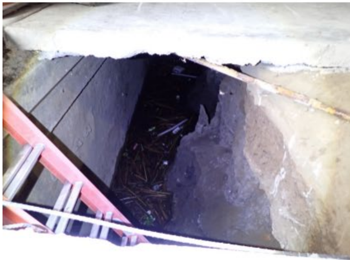
VOID EXTENDS FULL HEIGHT OF WALL NOTE WATER AND DEBRIS VISIBLE WATER LEVEL FLUCTUATES WITH TIDE
